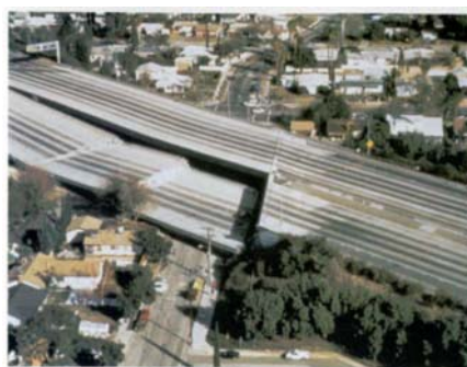
Collapsed section of I-10 (Santa Monica freeway), West Los Angeles. The freeway had been built across relatively soft soils (drained wetlands), the probable reason for the structural failure. This section of freeway was repaired and made serviceable in three months time. Photograph by Kerry Sieh.
